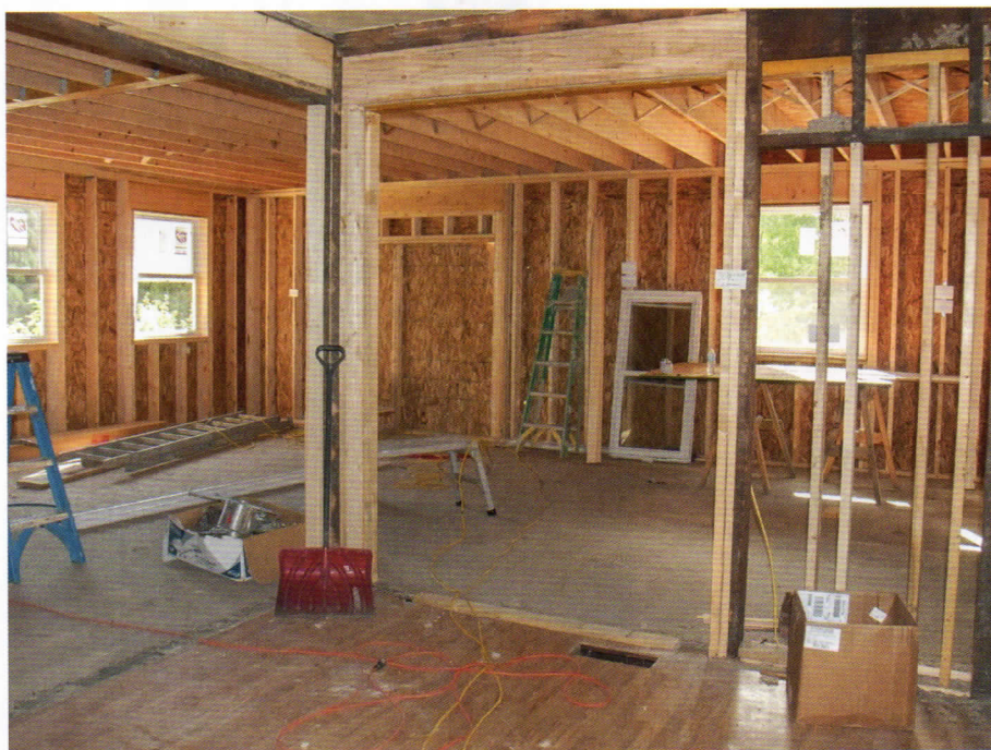
TOP: A major project can hugely enlarge and improve a bungalow. A dormer conversion and new roof by Trussty Loft Conversions at 07809 467644. ABOVE: Prepare for disruption but it can be worth it.
